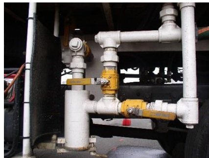
Material supply 'whitey' valves.
