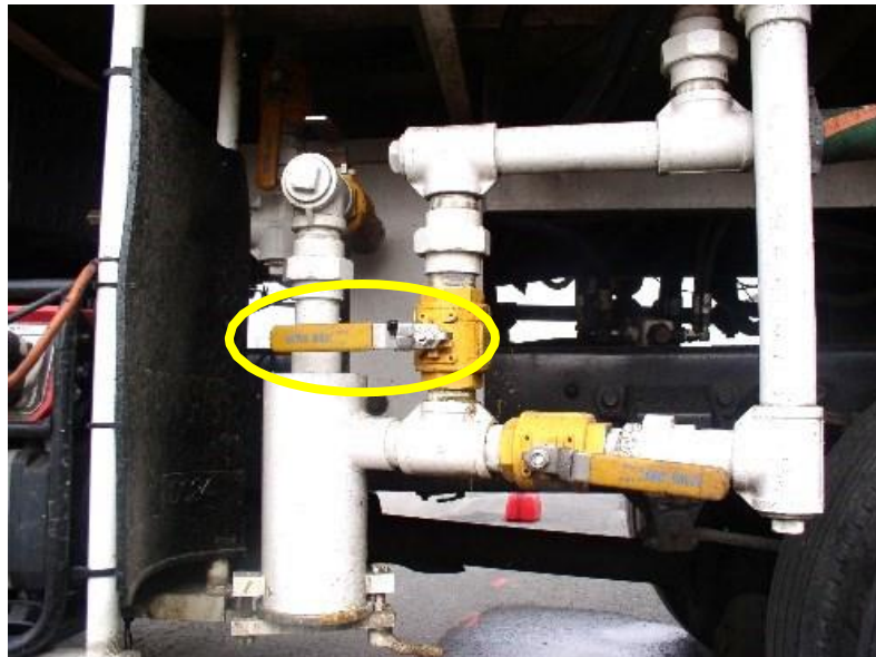
Heat Exchanger Bypass Valve (Closed)
